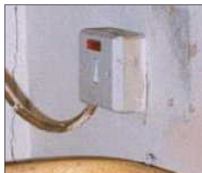
Switch to immersion heater
