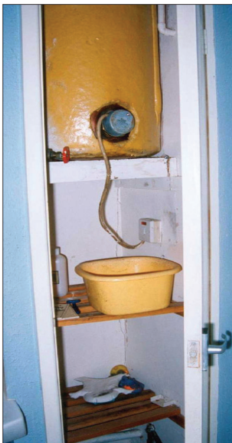
Airing cupboard with hot water tank above
